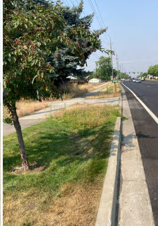
Curb and sidewalk at 3050 Prairie Ave.
