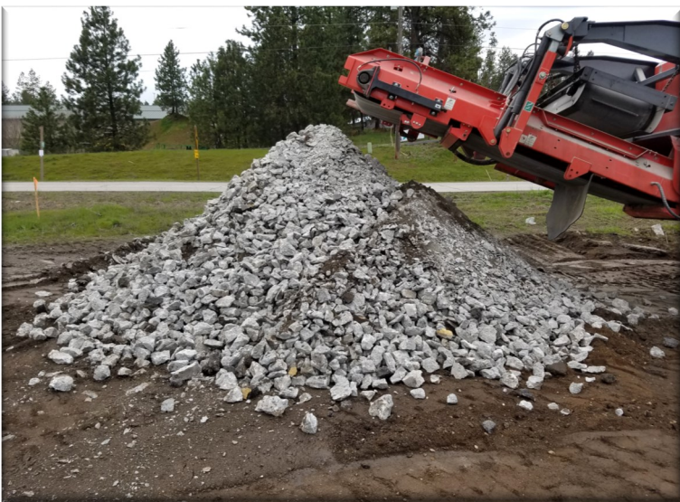
Concrete crusher "The Jaw" processing the 1940's roadway. Material will be recycled and used in the new road.
