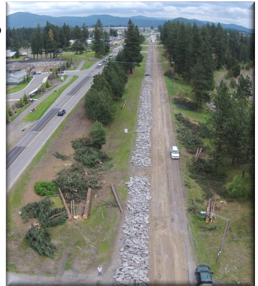
Eastbound lanes and select tree removal making way for new Seltice Way.
