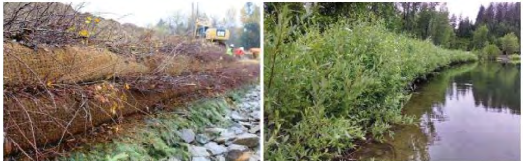
Before and after: The left photo shows the soil burrito in progress at the Kahnderosa Campground. The right photo shows how a previous installation at Medimont, Idaho turned out.
