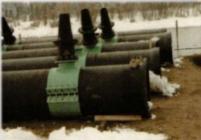
OUTFALL PIPE & DISCHARGE PORTS
