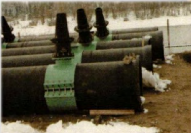
OUTFALL PIPE & DISCHARGE PORTS
