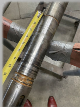
DAMAGE TO SHAFT
