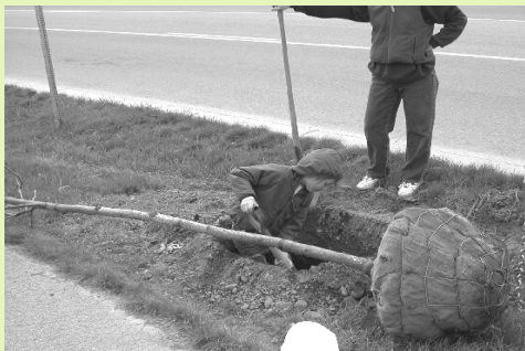
Don't worry about getting 'stuck in a hole'. Contract crews will do the tree planting!
